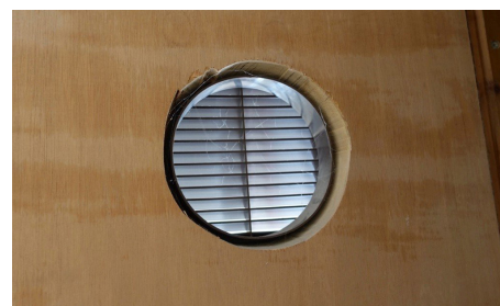
The fire door has had changes made to it after it was fitted, for example a ventilation grill has been added.
