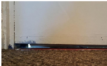
Fire door does not close properly or there is a large gap at the edges or underneath.
