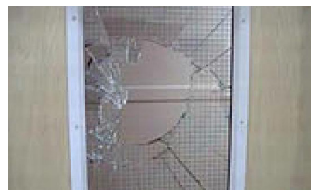
There is damage to the glass panel.
