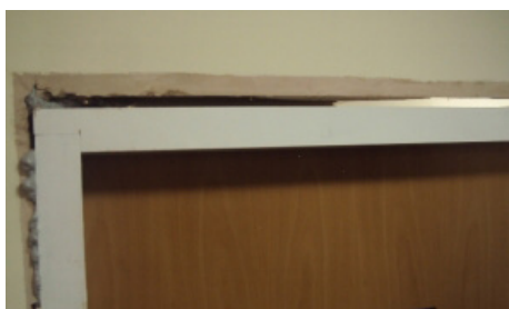
The fire door frame is damaged or poorly fitted.
